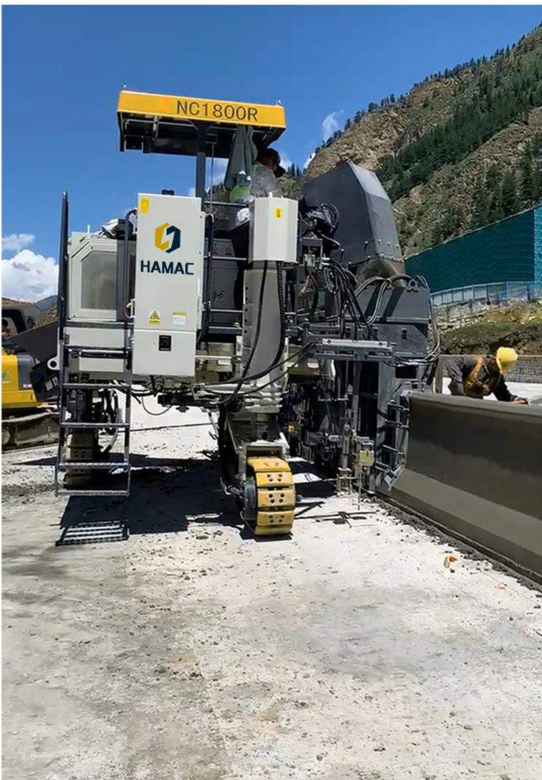
Slipform construction of anti-collision guardrail in Xining Hydropower Station No.15, Qinghai Province
