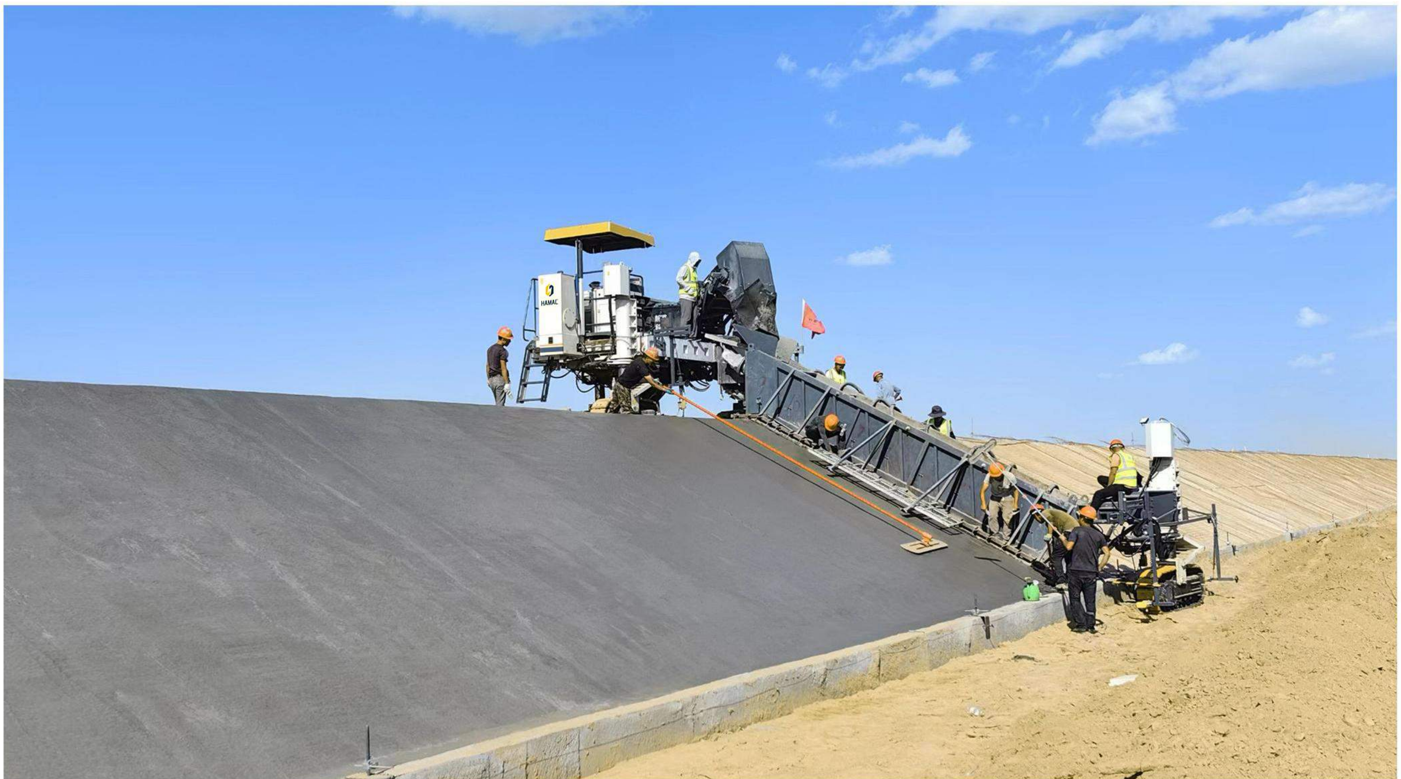
Sliding form construction of 6-meter wide slope protection in Linhe District, Bayannur City, Inner Mongolia Autonomous Region
