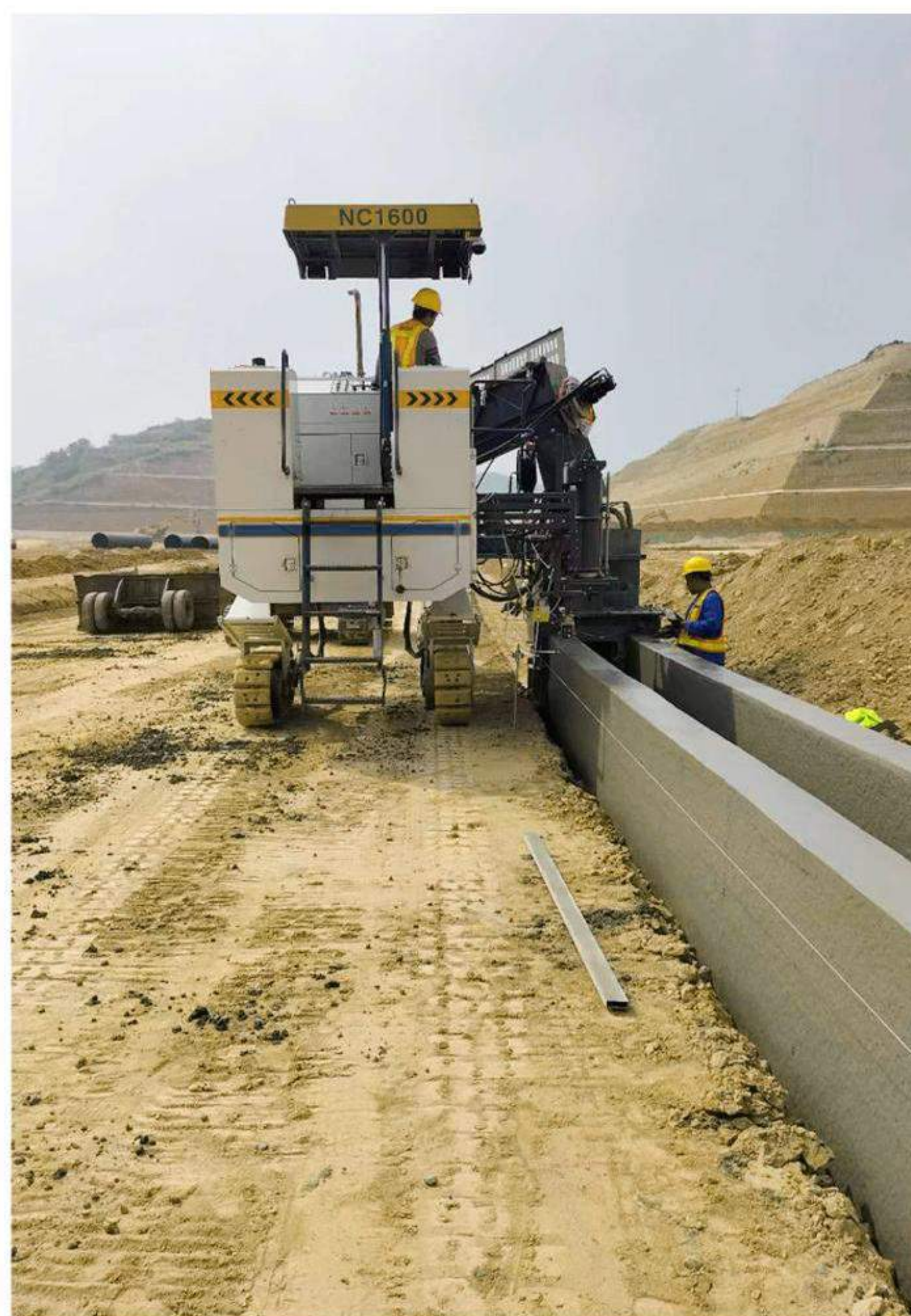
Sliding form construction of drainage ditch in Jiaokou County, Luliang City, Shanxi Province
