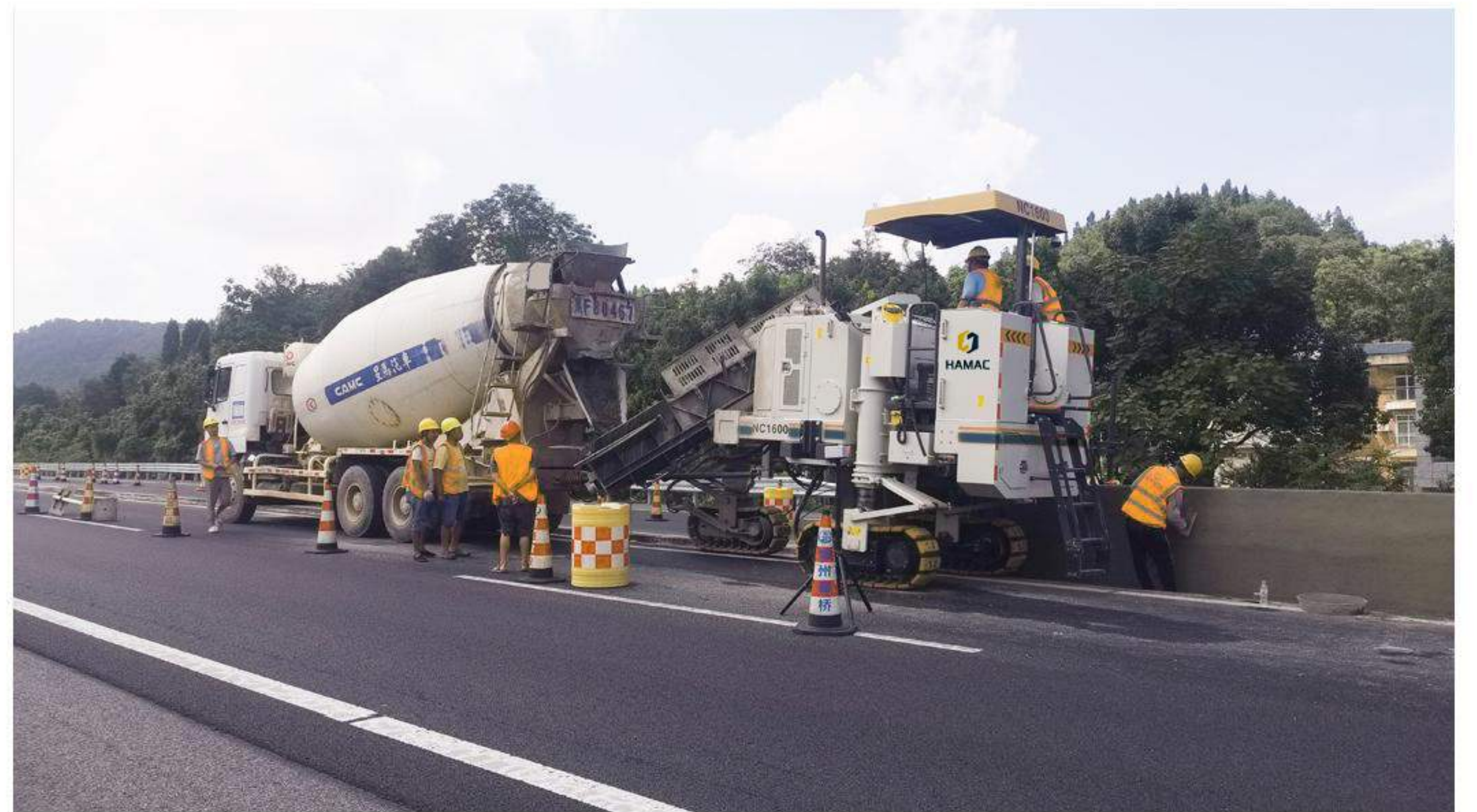
Sliding form construction of anti-collision guardrails in Sansui County, Qiandongnan Miao and Dong Autonomous Prefecture, Guizhou
