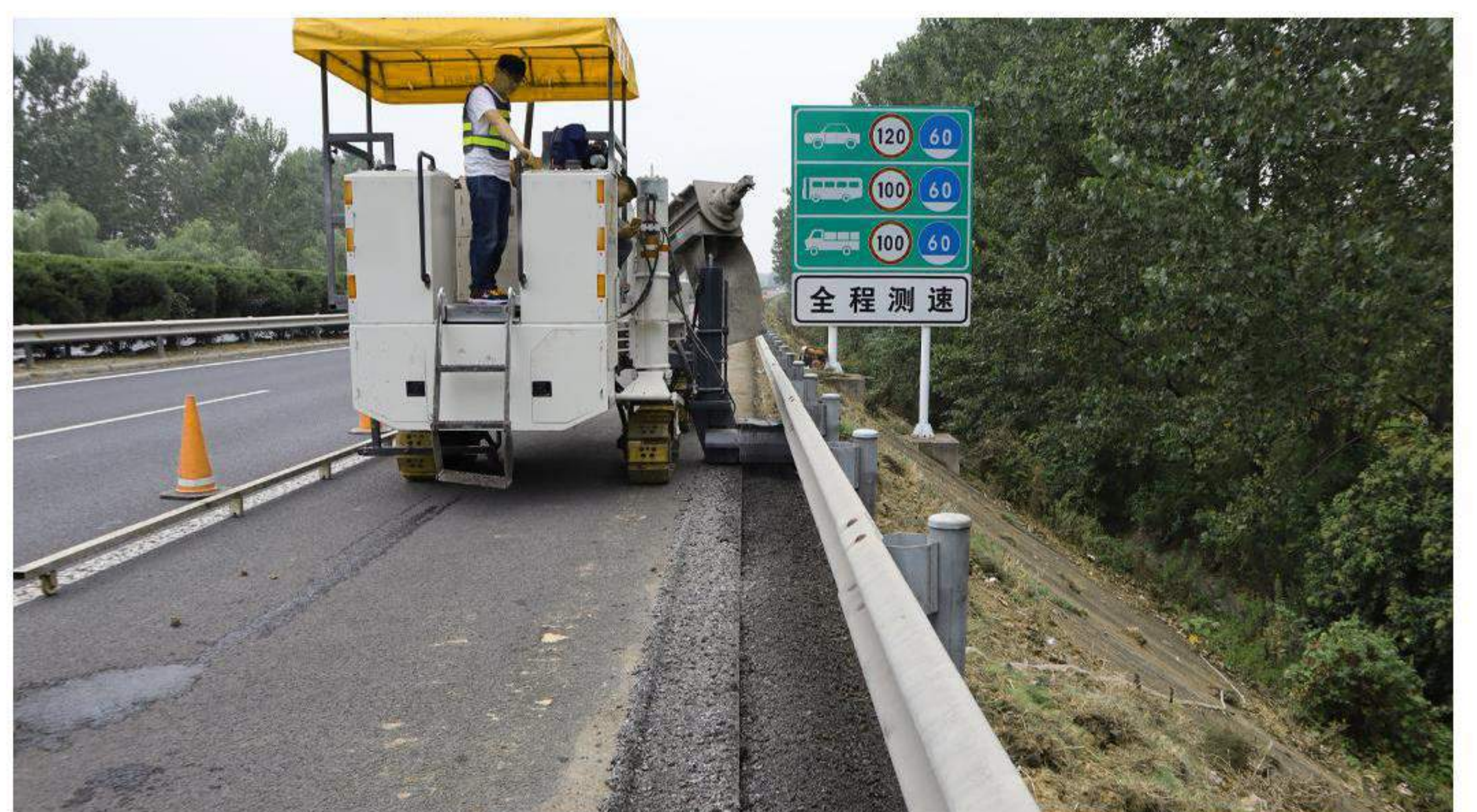
Slipform construction of high-speed lateral milling and planing and butterfly-shaped side ditch in Suhuiyan
