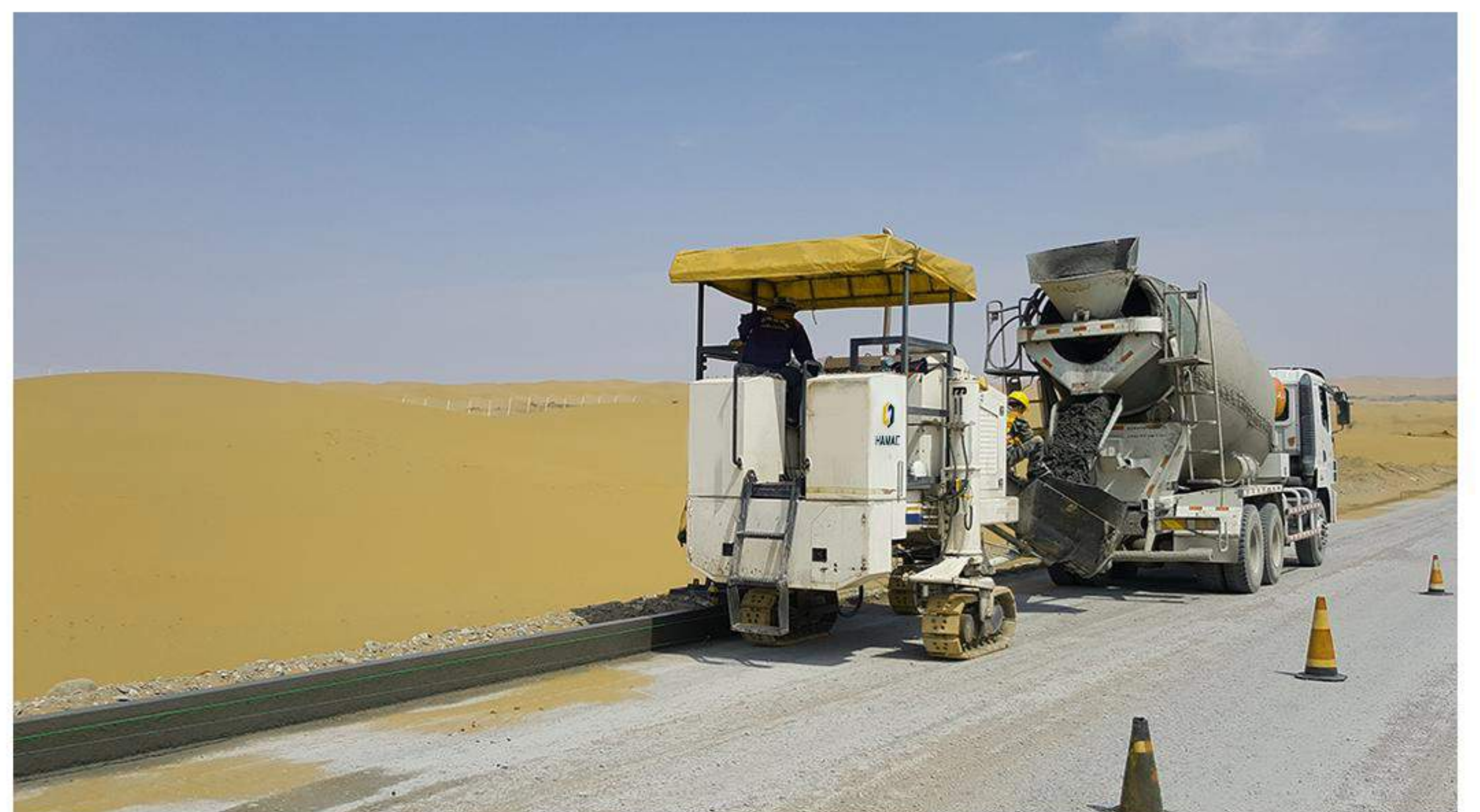
Slipform Construction of Curb Stone in Dream Park of Alxa League, Inner Mongolia
