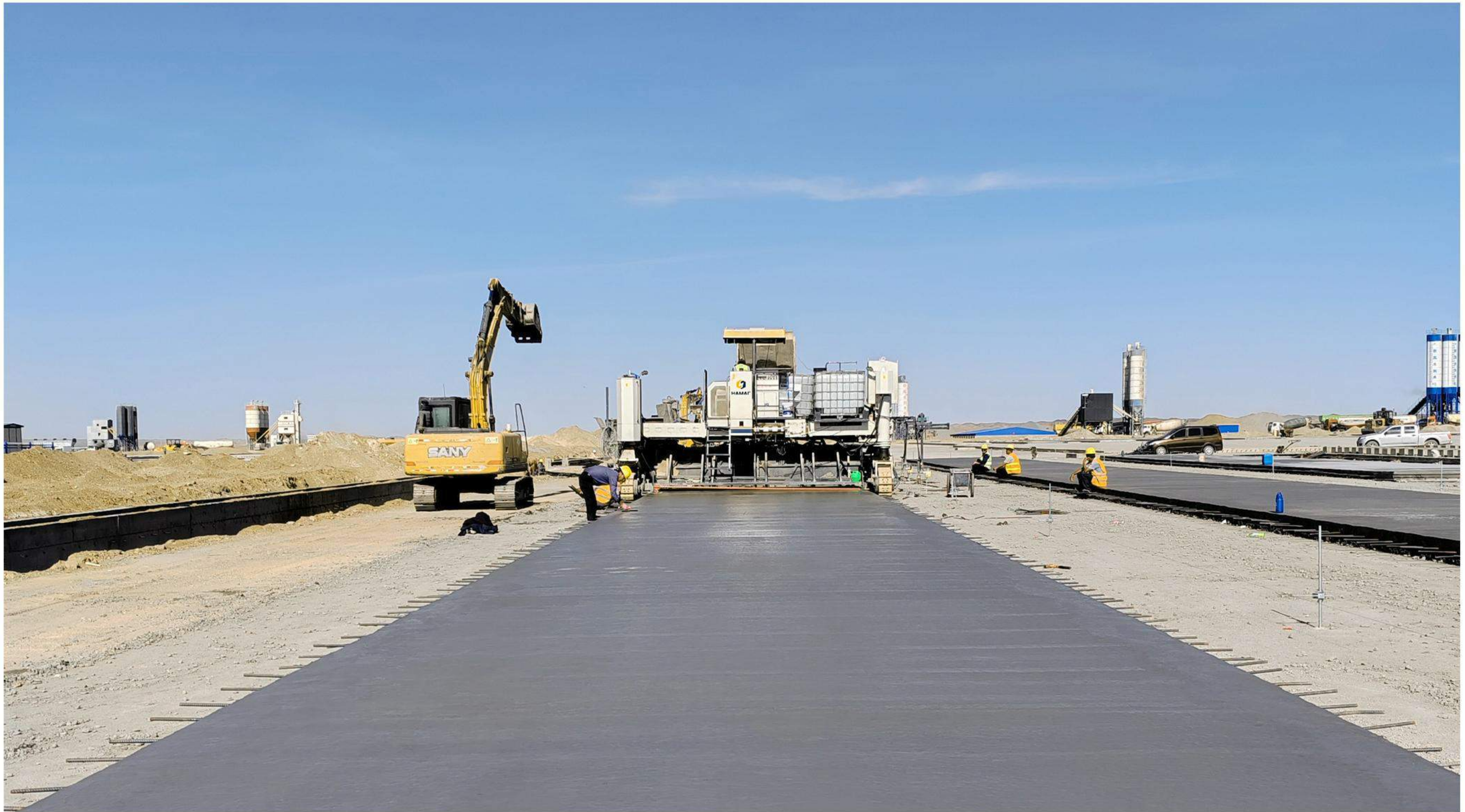
5-meter wide road paving construction at Ganqimaodu Port in Inner Mongolia Autonomous Region
