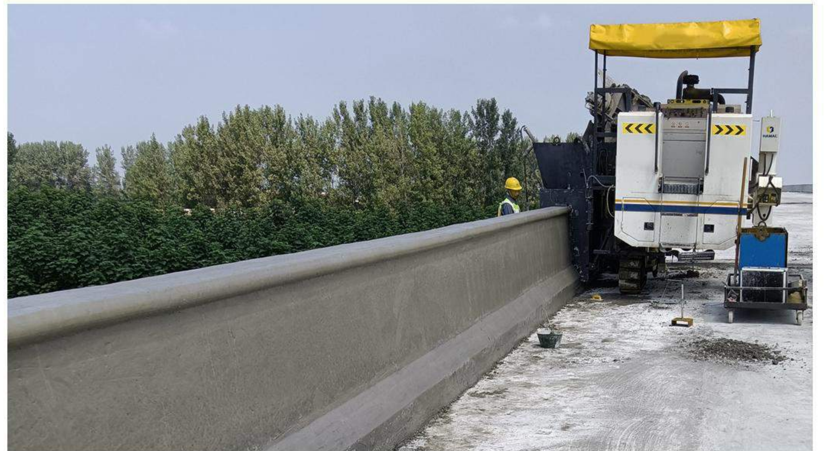
Sliding mode construction of anti-collision guardrail of Luohe bridge in Henan Province
